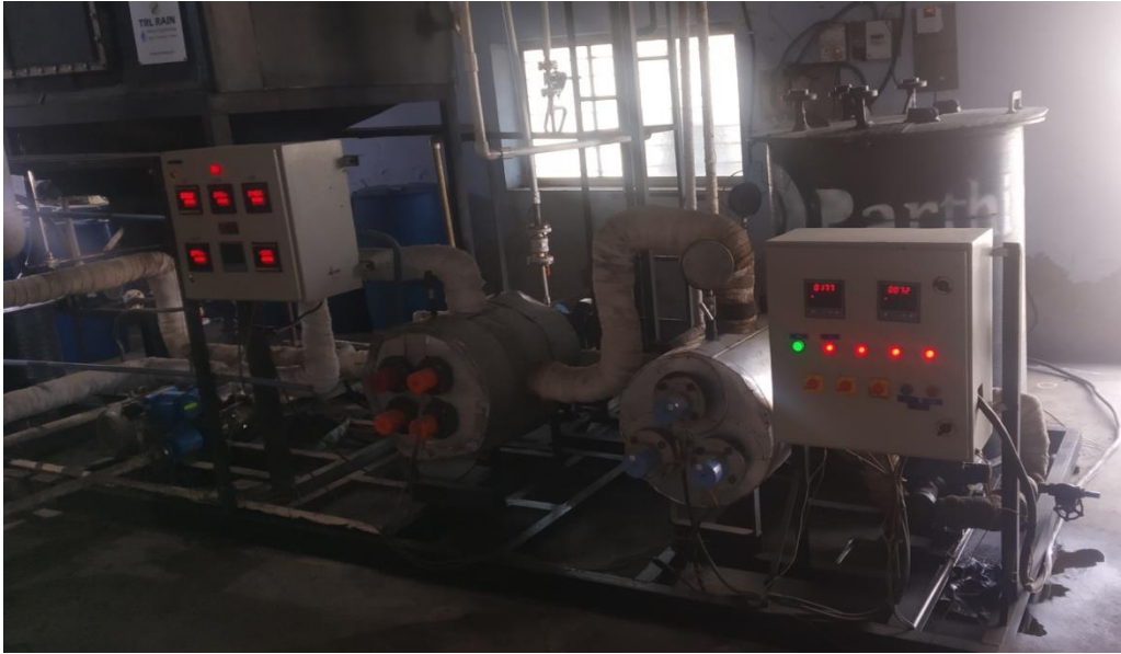
Thermic Fluid Heater
